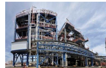
Polycarbonate diol (PCD) manufacturing facilities (Spain)
