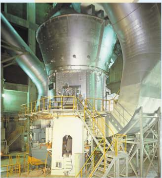
Vertical mill (Industrial machinery)
